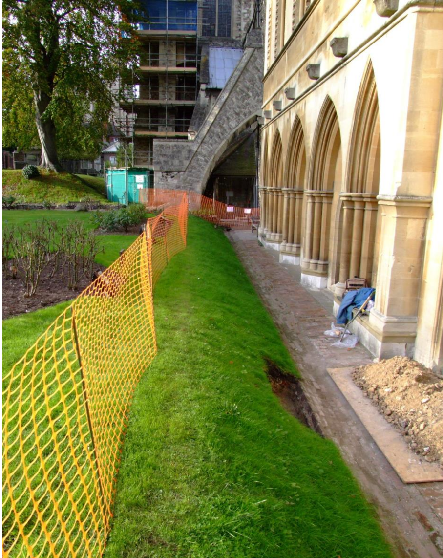
View along the north cloister walk at Rochester Cathedral in October 2007, with the South Transept shrouded in scaffolding.
