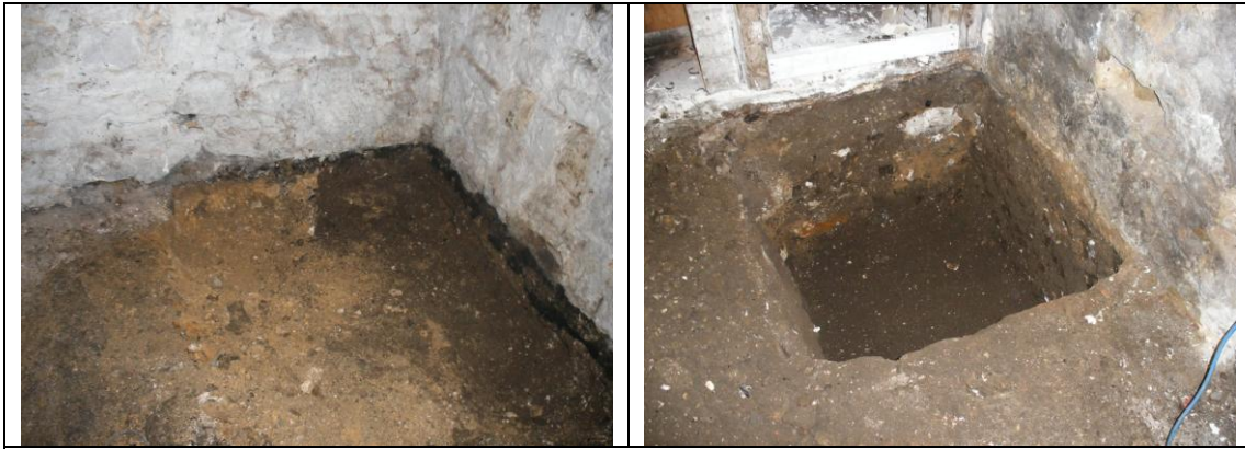
Figure 8: The basement test pits – left, pit 3, showing the gravel foundation of Deanery Gate and soil to the west (right) of it where the house extends beyond the gate; right, pit 2, with poorly differentiated soils under the east wall and floor.
