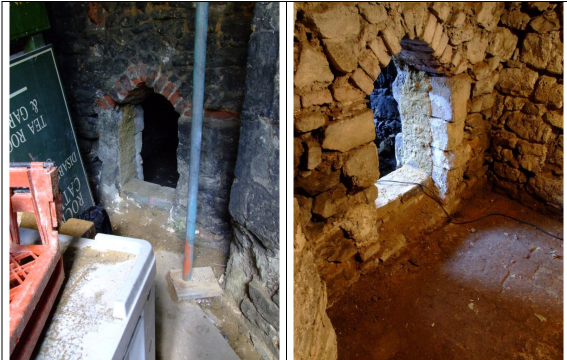
Figure 11: The unblocked door in the cross-wall from the outside (east) on the left, and inside on the right. Note the brick paving in the right-hand photograph.
