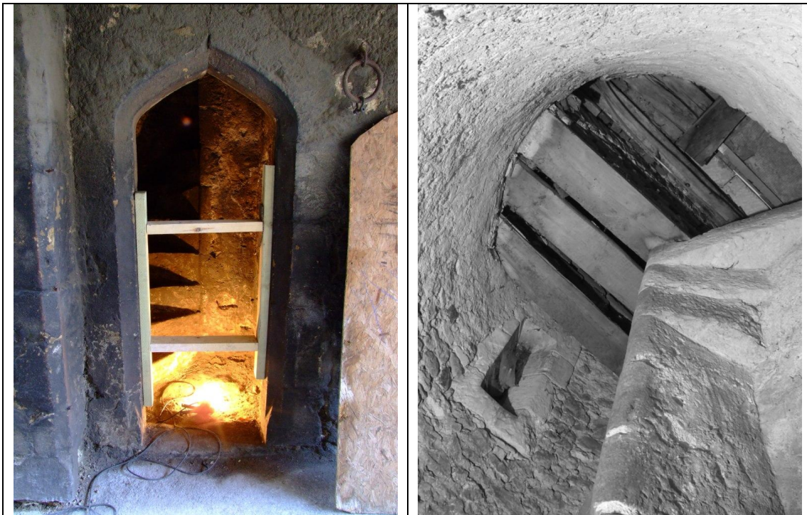
Figure 10: The newly unblocked door to the spiral staircase (left), with the slit window and the boarding under the fireplace in the upper chamber (right).
