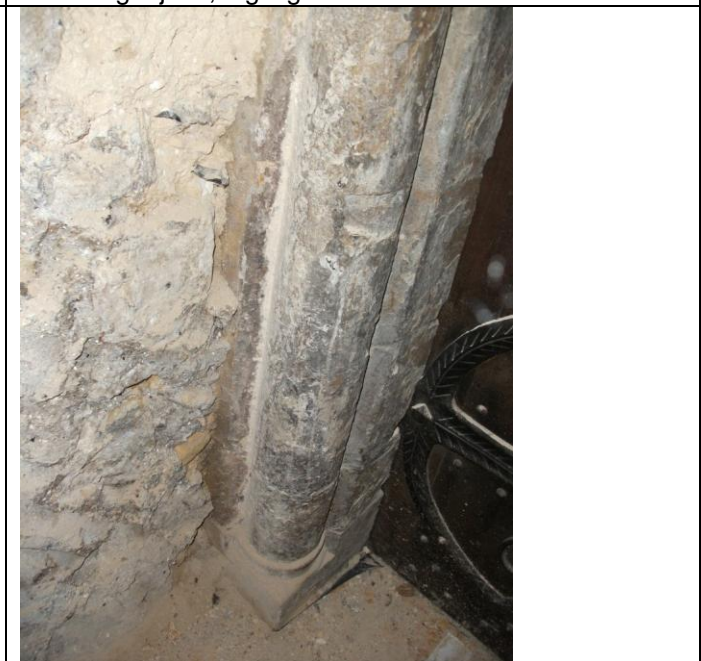
Figure 7: Abutment of the south wall with the door jamb of the West Front's south-west turret.
