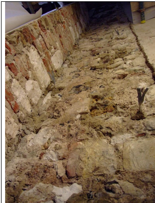
Figure 8: The pilaster buttress (left) abutting the masonry of the south wall. Note the frequent use of brick in both, but especially in the buttress.
