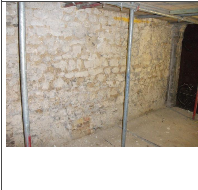
Figure 6: The remainder of the westernmost bay of the Nave south aisle. Most of this is 12 th -century fabric.
