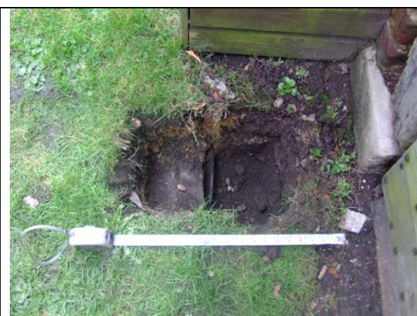
Figure 4b: Test pit 2 from the north with the feeder pillar behind it, 0.5m scale.
