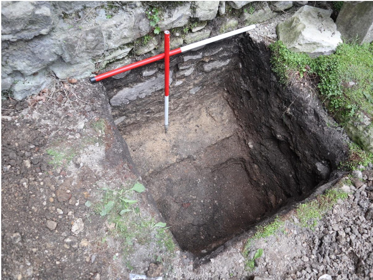
Figure 6: Pit 4 looking south-west, with the offset foundation plainly visible – note the slight upstand at its west (right) end. This image also shows the sondage dug in context 38/39 , in the lower right corner of the pit.
