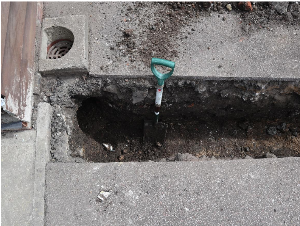
Figure 8: Sample section of the water main trench with rubble layer 18 at the base.
