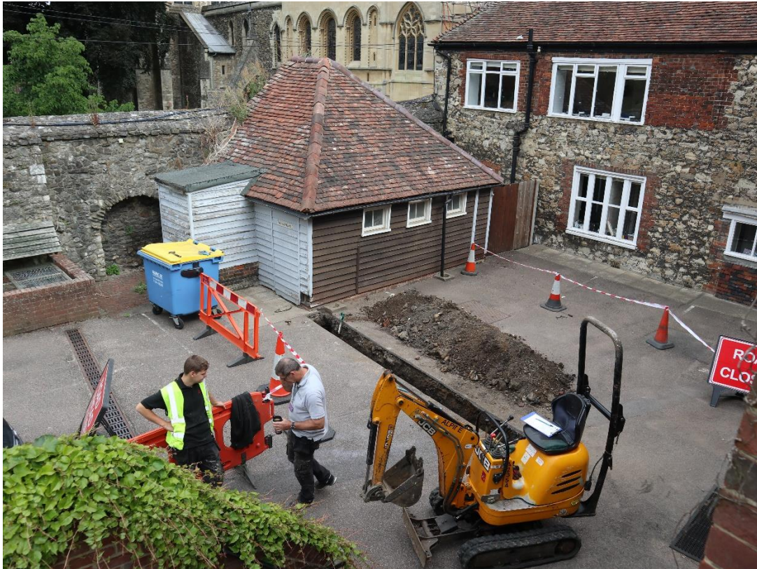
Figure 7: The new water trench in the former Dorter area, looking north-west. The stone range to the right is described as having 16 th -century rectangular brick dressed window openings in the listing, which would suggest a potential medieval date for the surrounding masonry (see footnote 1).
