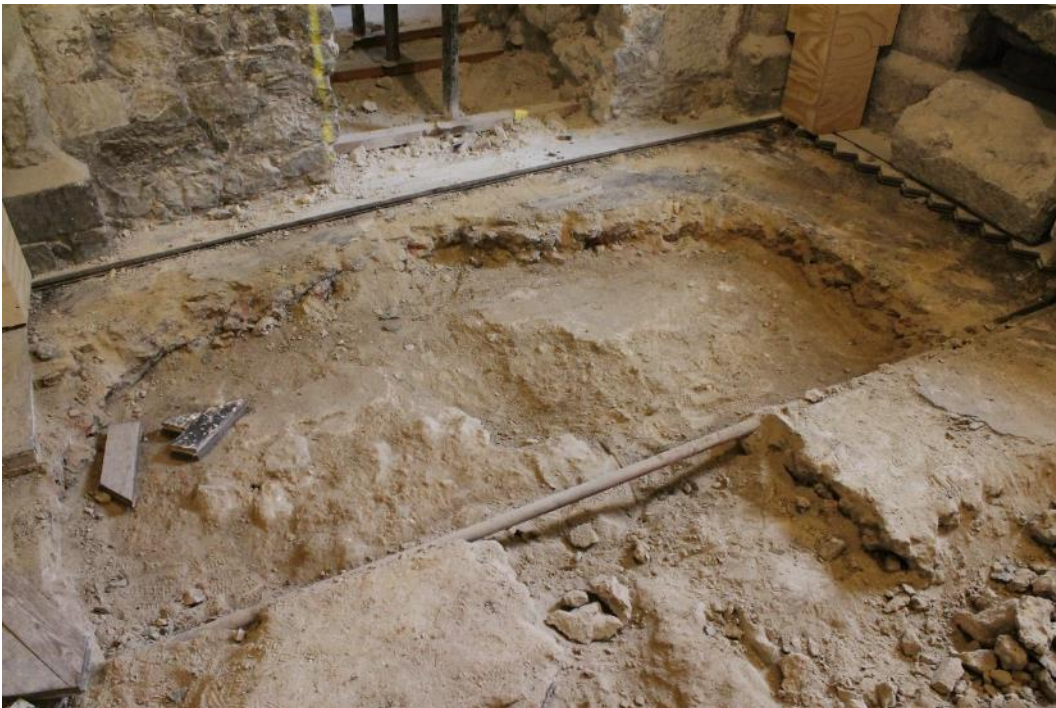
Plate 24: The south-east corner of the Norman foundations and buttress 1803 during initial cleaning. The straight edge of the south wall can be seen passing under the modern pipe.
