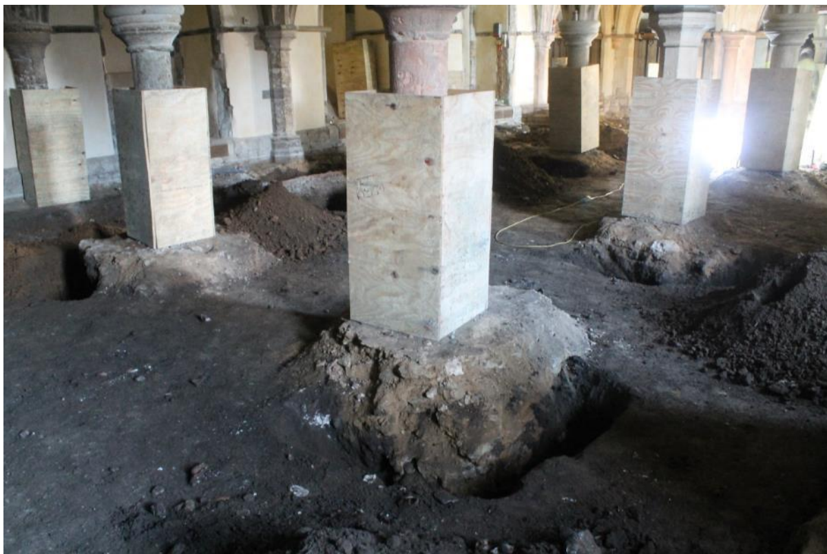
Plate 16: Excavation within St Ithamar's Chapel looking south-west, with the dark brown clayey loam exposed between (and cut by) the late 12 th -century foundations for the chapel vault.
