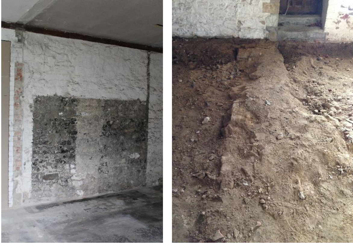
Plate 39: Left – the scar of wall 1160 in September 2014 after the vestry had been stripped out (the below-ground works would wait for another year, so the foundation was only exposed then). Right – foundation 1159 abutting the south wall of the vestry.
