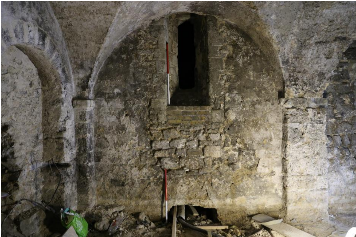
Plate 18: The partially blocked arch in the outer wall of Norman crypt's north aisle was used as the route to get the new heating ducts from under the crypt floors into the 'Gundulf Shaft' behind the arch. The area of blocking between the two 1m scales is easily recognisable on the left (west) side of the arch in this photograph, taken just before work started in June 2017.
