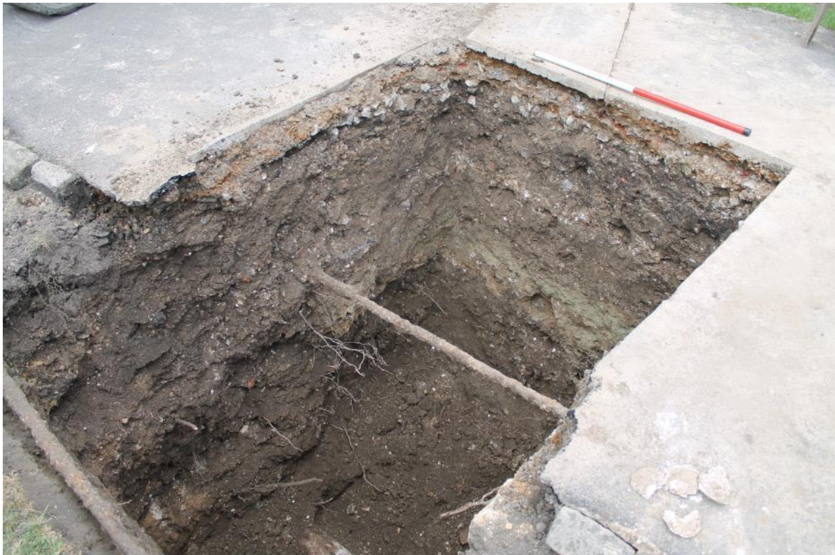
Plate 9: The excavation for a new manhole in the roadway, with the existing sewer just visible at the bottom, looking north-west. The edge of the pipe trench can be seen quite clearly in the long section, cutting through all the layers except for the tarmac and its bedding.
