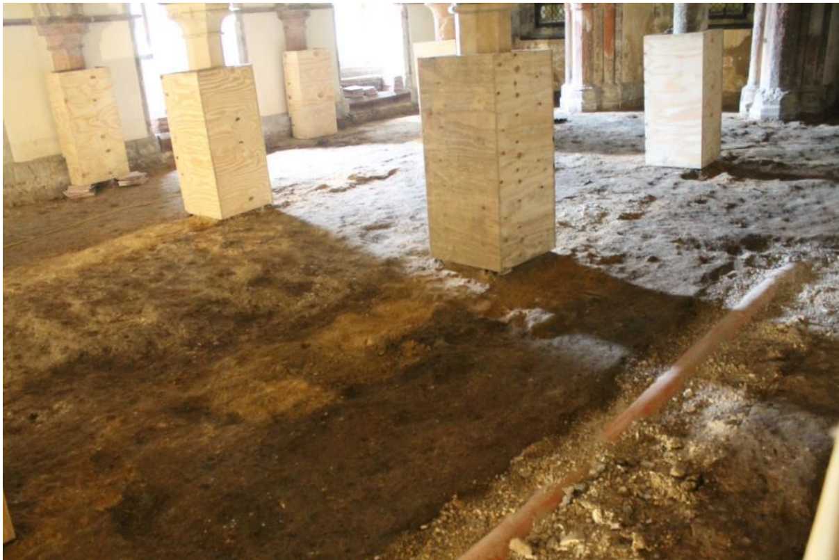
Plate 17: Excavations in St Ithamar's Chapel at an early stage, with the foundations for the High Altar support walls (615) and patches of mortar floor/bedding (605) exposed.
