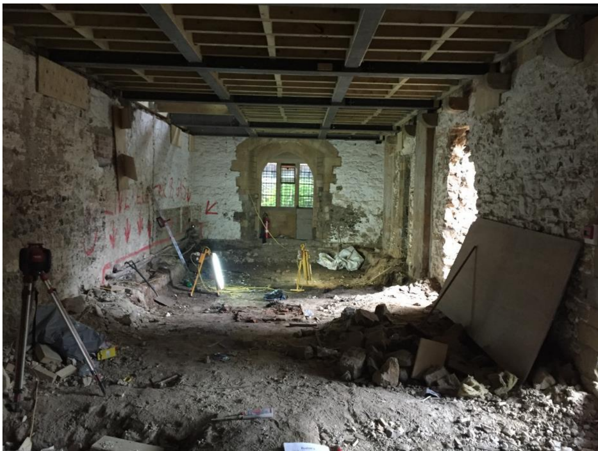
Plate 36: The vestry off the south-east corner of the main crypt under excavation in October 2015. The wall bench can be seen in the background, with tiled hearth 1111 in the centre of the room.
