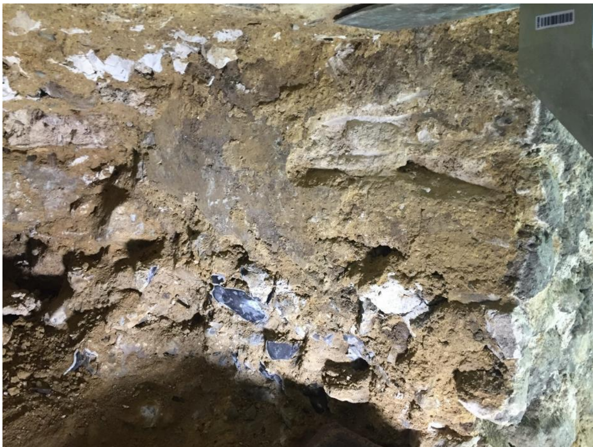
Plate 19: The tufa jamb stones on the east side of the arch were exposed during the work. The area of render in the centre of this photograph is original, ie Norman. The blocking of the arch, though all but solid, peeled away from the render surprisingly easily.
