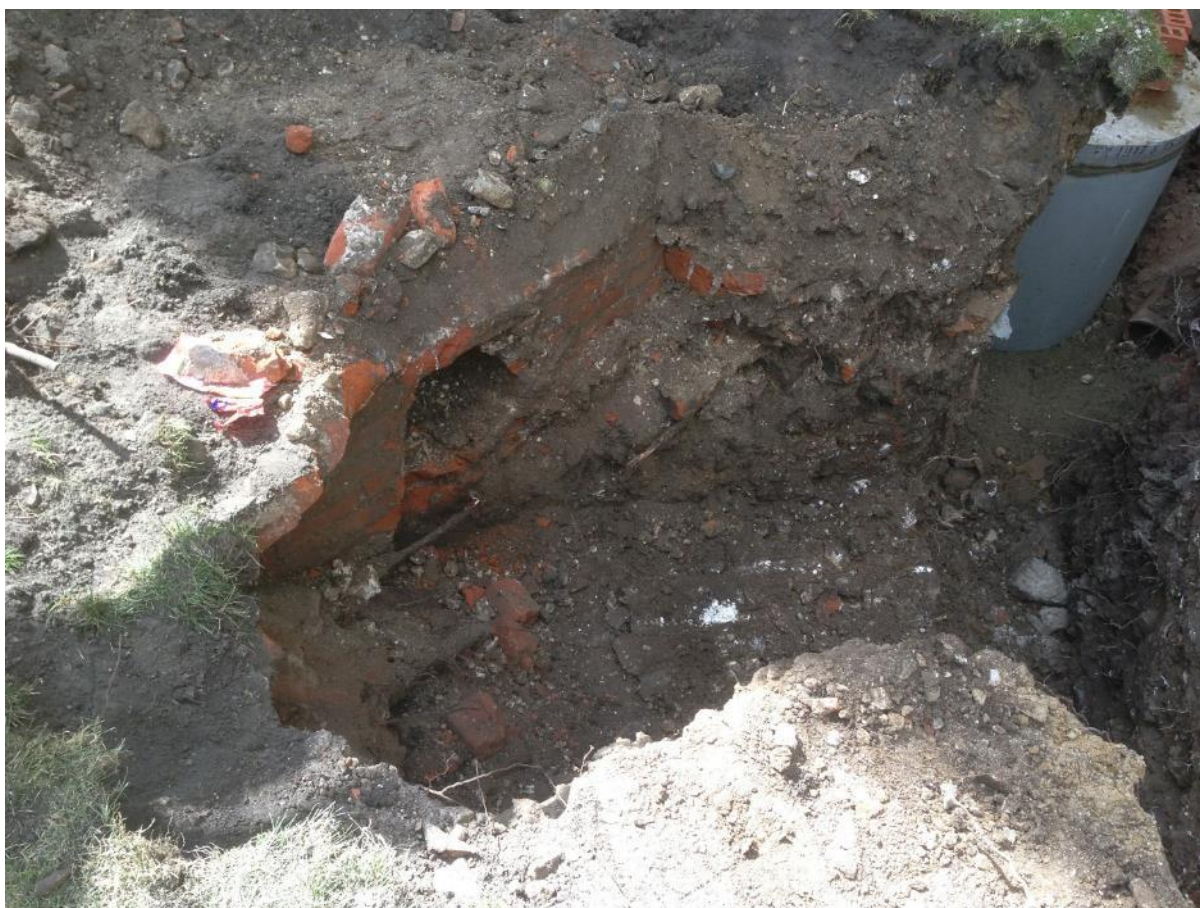
Plate 10: The remnants of culvert 27, with the opening for the adjoining culvert 28 visible.
