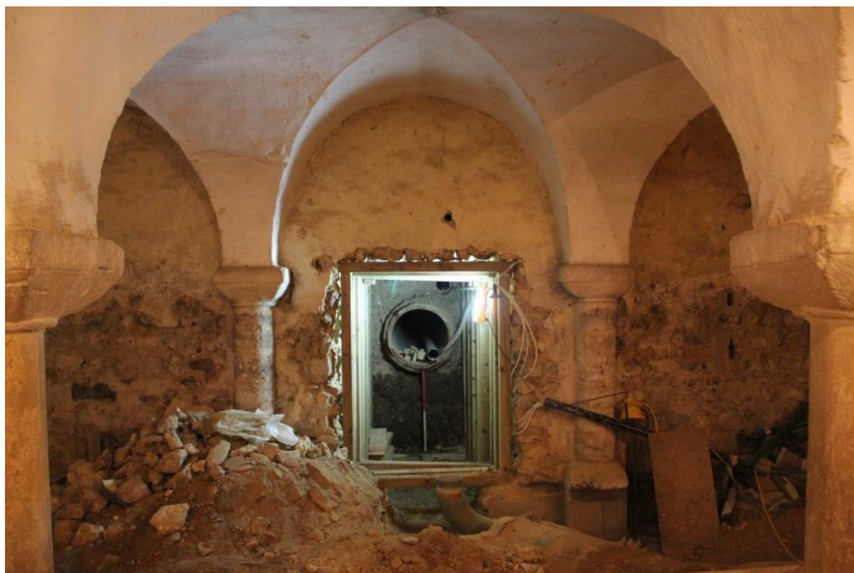
Plate 12: Irvine's tunnel being re-excavated, January 2016. The 1m scale rests against Roman layer 1226, which Irvine had left largely in situ - the grey backfill of his trench is clearly visible above it.
