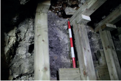
Norman floor ('roof' of the tunnel) at the top, and the dumped layers under it in the side/section.
