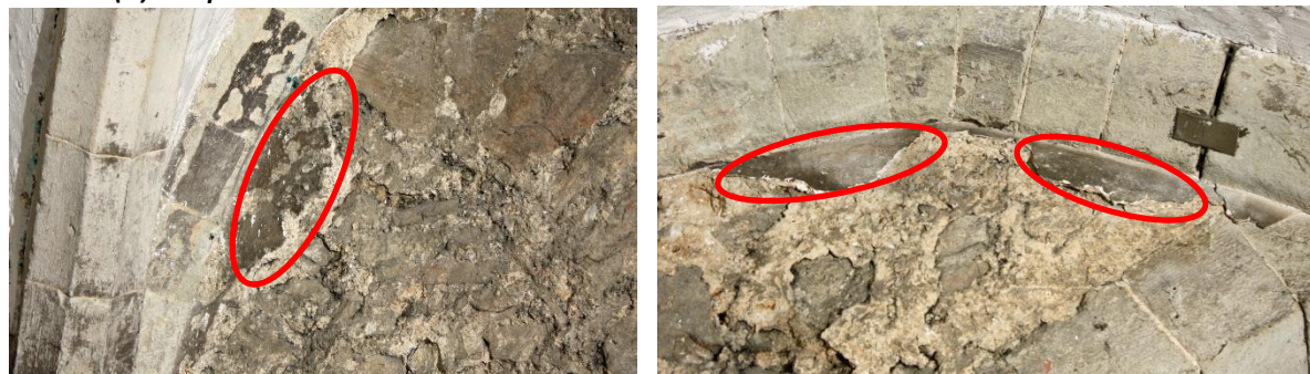
Fig 1. Islands of plaster and unpainted early-limewash on Bay 19 , north wall before dusting and plaster edge repairs. It has not been established if the red ochre masonry line paint exists on these fragments. (A) samples (2 x limewash, 2 x paint(?)) = 4 (A) samples (max) .
