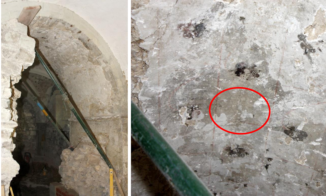
Fig 2. Recently revealed painted plaster on the arch soffit between Bays 13 and 20. This area had been blocked in since 1776-78. The whole soffit is untreated but the discoloured patches more closely resemble pre-treatment Phase 1 surfaces. (A) samples (2 x limewash, 2 x paint) = 4 (A) samples.
