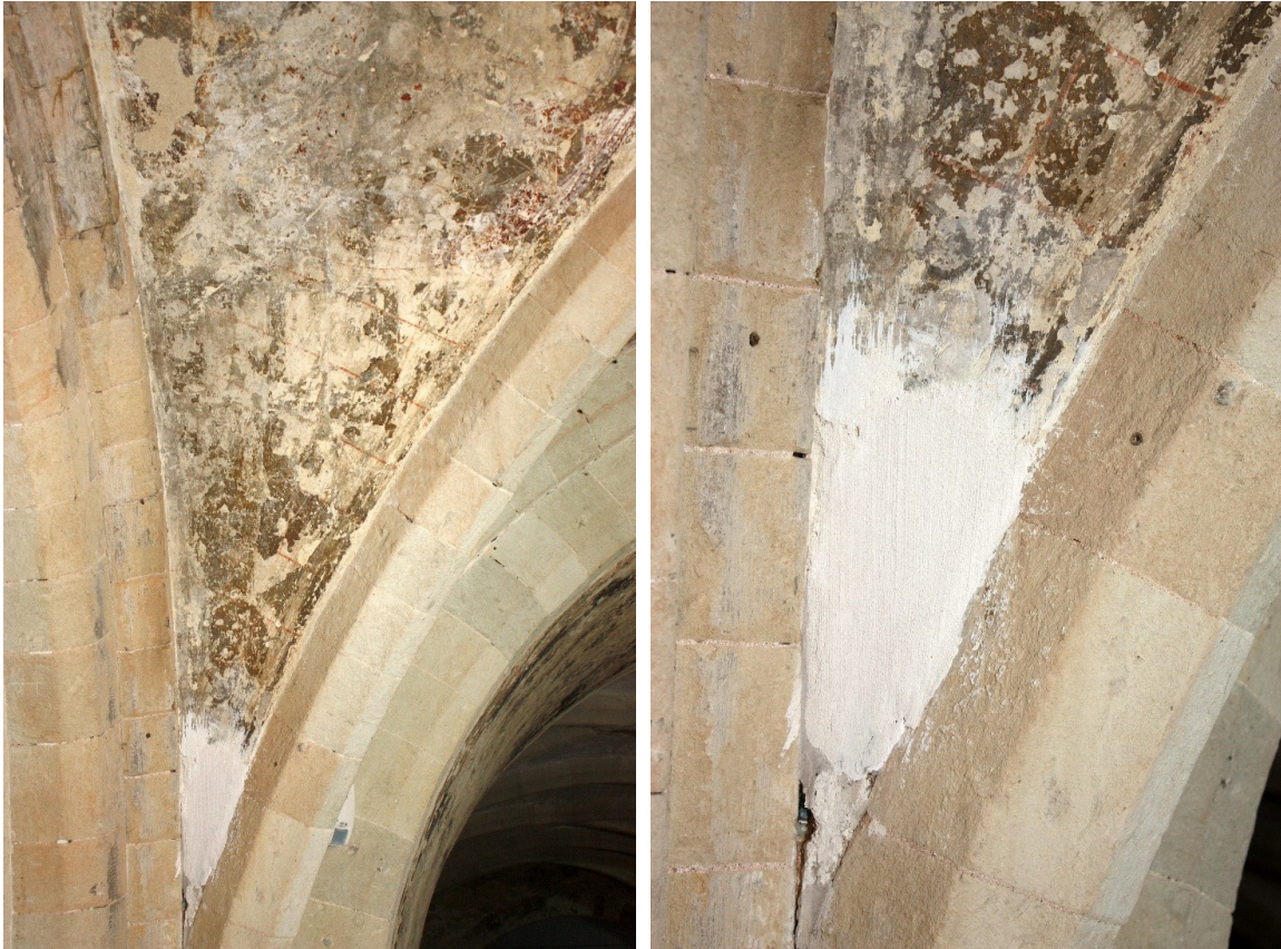
Fig 3. (above) An inappropriate plaster repair to Bay18b 2 inserted during the recent Crypt renovation works should be replaced and toned in to match other repair plaster in this vault.
