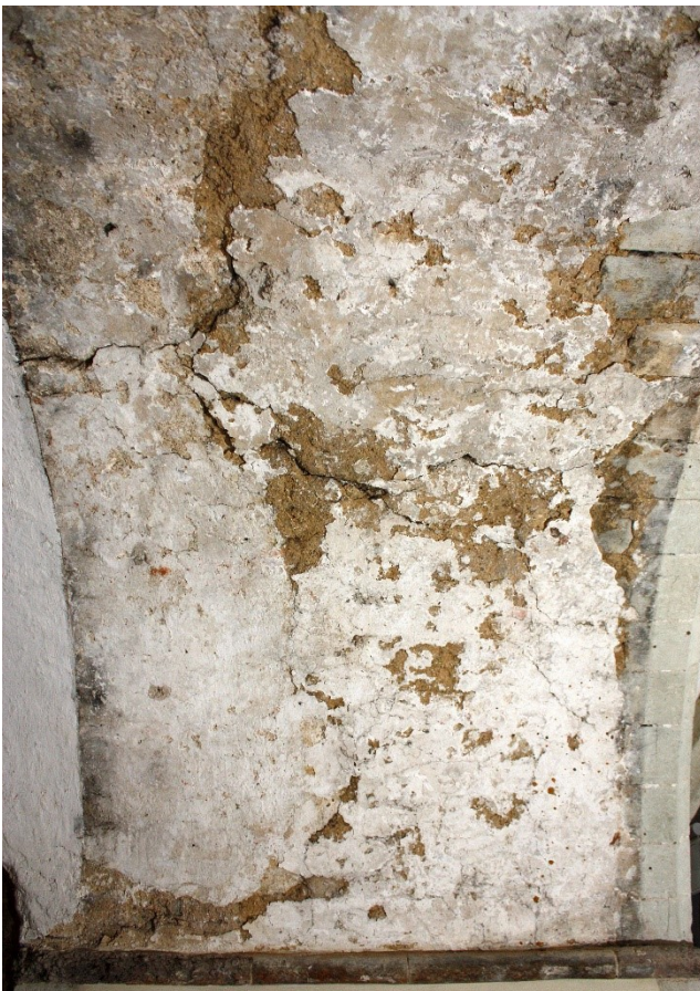
Fig 6. (right and below) Soffit of the arch between vault Bays 49 and 35. This area of original plaster, limewash ground and traces of painted decoration was revealed when the brickwork infill was removed from this archway. Traces only remain of painted decoration on the limewash ground which itself has suffered considerable damage and loss: as has the surface plaster skim and the substrate plaster which in places is cracked, displaced and unstable.
