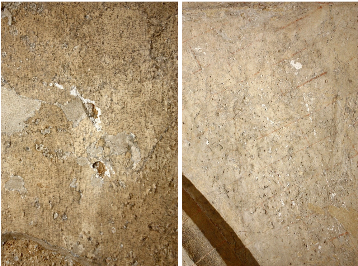
Fig 4. (above) Instances of recent indents, loss and scrapes to the plaster and ground of Area J and Bay 2a 1 .
